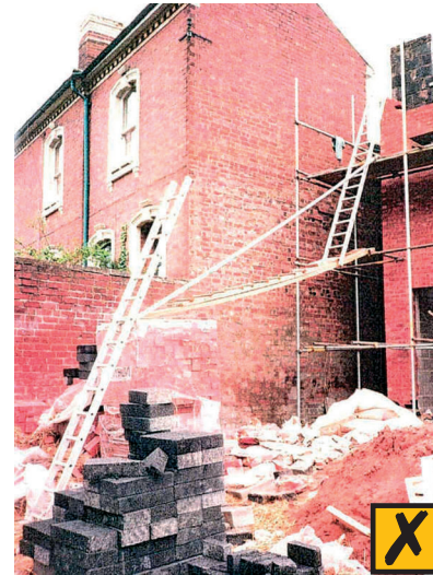
2.0 Highly dangerous practices involving the use of ladders.
